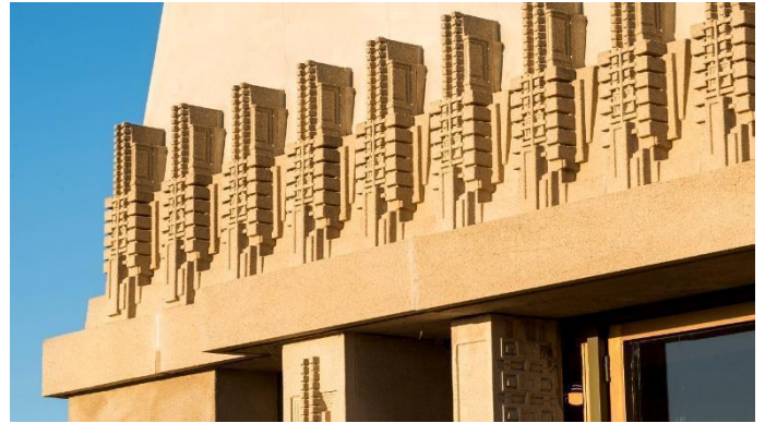
Detail of art stone on west façade, Hollyhock House. Joshua White/JWPictures.com, courtesy of Hollyhock House. DOWNLOAD THIS PHOTO
